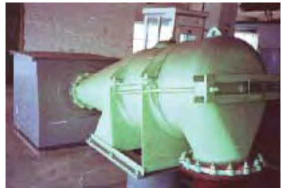
Heavy media cyclone
